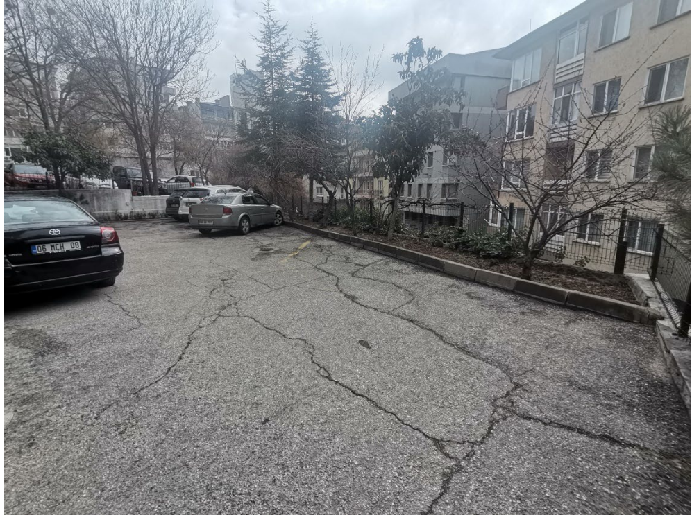
Figure 63. Existing condition of Patch 63.
